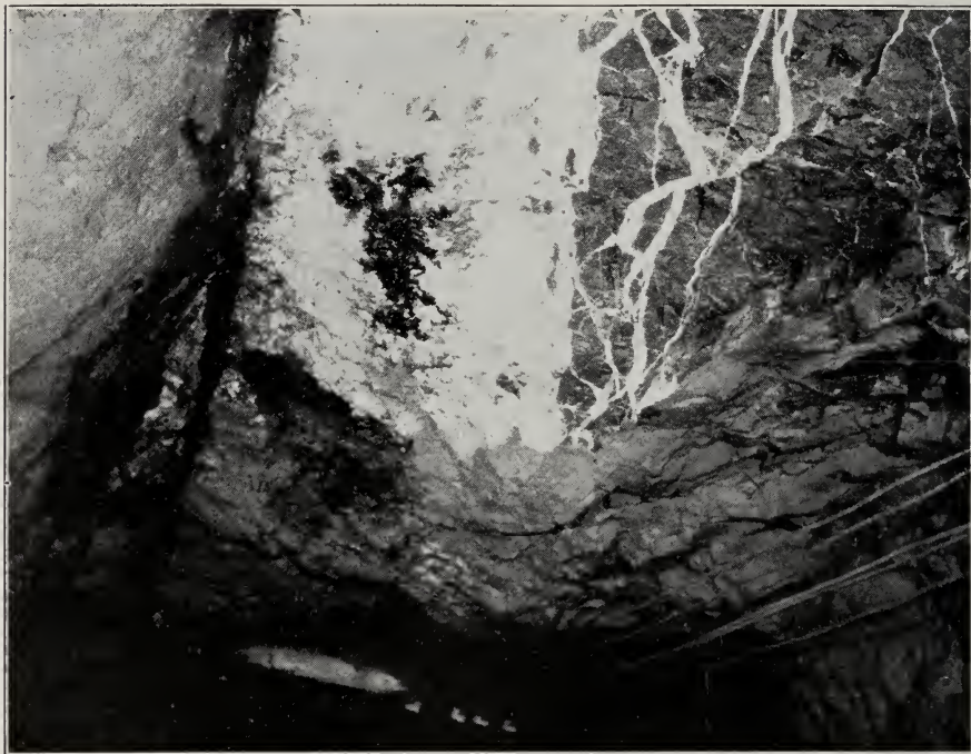
FIG. 3. Daisy vein, about 3 feet wide, in the top of the 412-foot level of the Daisy mine, looking north toward the main shaft from near cross-cut. The sharp contacts between the vein material, mainly calcite, and the limestone of the foot wall (right) and the angular, ragged limestone fragments in the vein are well shown. The hanging wall (left) is a smooth, slickensided surface along which there has been movement since the vein was formed. The irregular dark patch near the center of the vein is a stain produced by seepage of petroleum out of the vugs in the vein.
